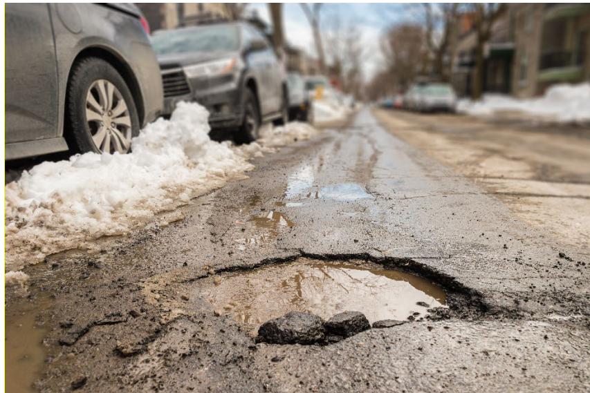
Pothole in Montreal. Image licensed from Adobe Stock.
