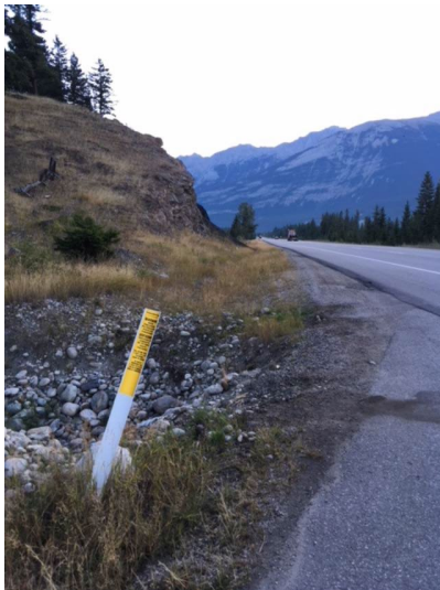
This is a picture of the completed Trans Mountain Pipeline, invisible once completed. Image courtesy Rob Pearce
