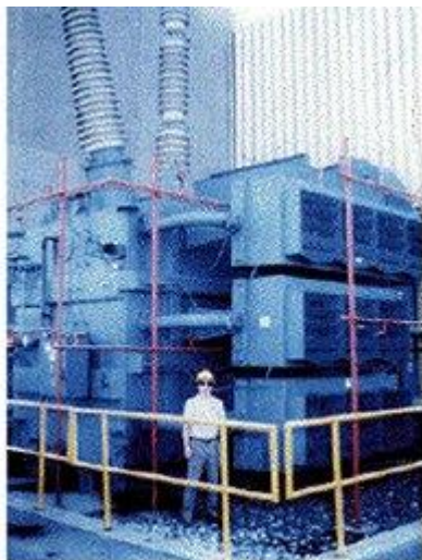
PJM Public Service Step Up Transformer
